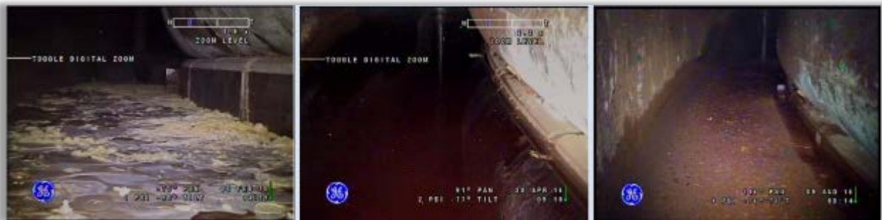
Figure 16. Annulus Waste Condition
